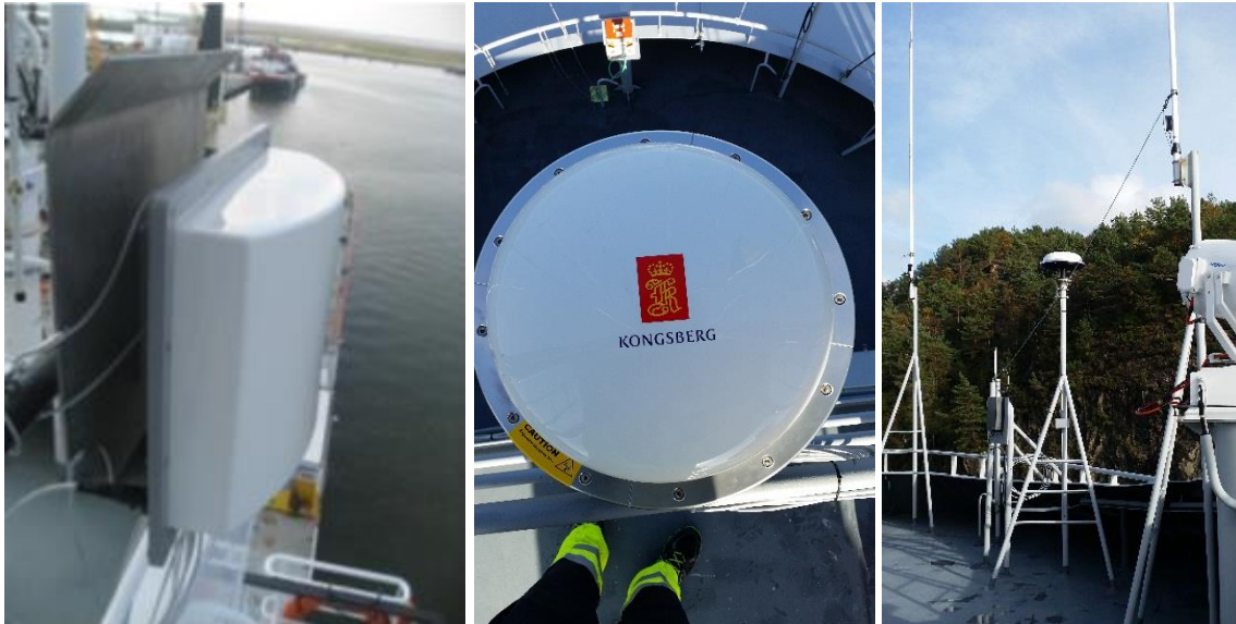
Figure 6: Example of MBR installations on board a vessel
