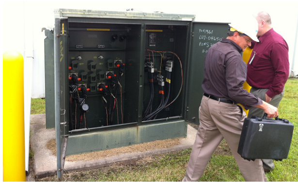
Figure 3. 6.8 kV pad mount transformer with wireless sensors installed.
