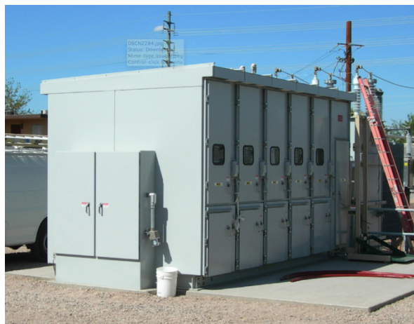
Figure 4. A small bank of medium voltage switchboxes shows both weather-tight and RF-tight enclosures. Such systems have very low spurious emissions.
