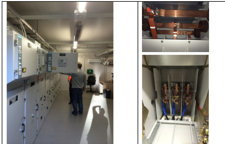
Figure 6 shows that indoor medium voltage switchgear, such as these Siemens 8BT1-24 operated by a utility in Finland, employ multiple layers of steel construction between the positions where antennas and sensors would be located and the interior of the structure housing the switches.
