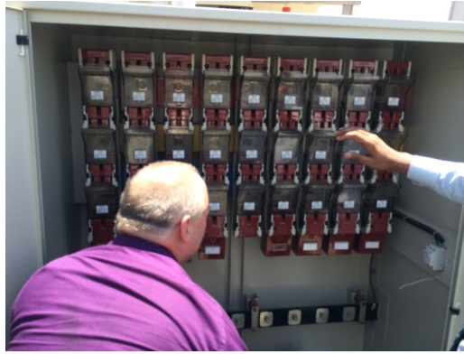
Figure 7 shows a low voltage distribution panel in a typical metal cabinet.
