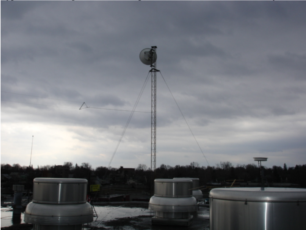
Typical Test Configuration – Existing mast on the roof of 1680 University
