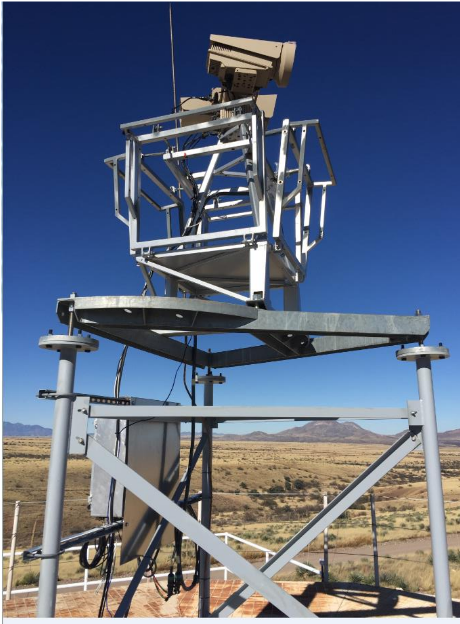
Figure 3 – Radar Mounting Structure – Fort Worth, Tx
