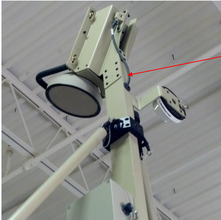
Figure 74. Lightning Grounding Cable
