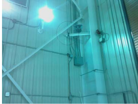
Figure 10: IPF Interior Antenna
