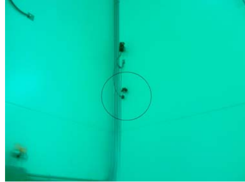
Figure 6: PPF Interior Antenna 2
