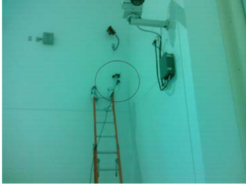
Figure 5: PPF Interior Antenna 1
