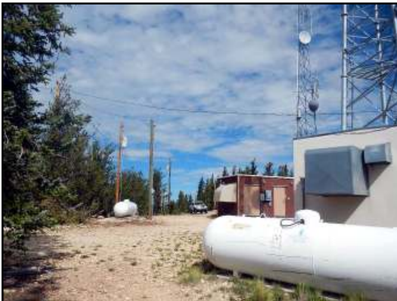
Photo No. 2. Looking north over the surveyed area on Green Mountain. Existing utility poles and equipment associated with standing telecommunications towers are visible in the photo.
