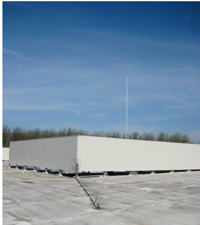
Figure 6: The outdoor rooftop antenna structure in a planned test site.
