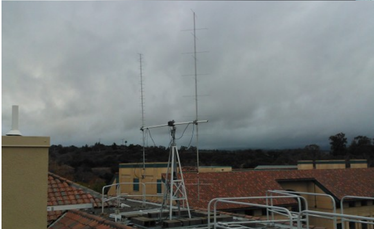
Figure 3 UHF/VHF Antenna on Durand Building Roof
