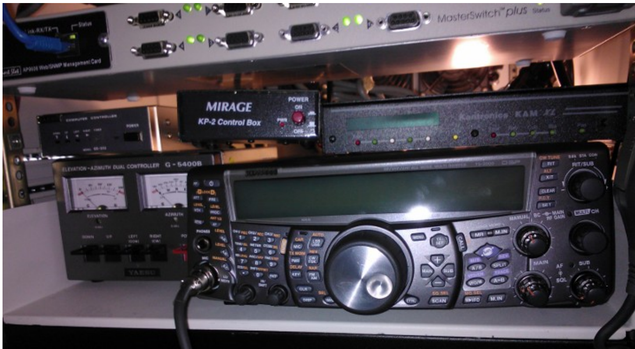
Figure 2 TS-2000 Transceiver in SSDL Ground Control Room
