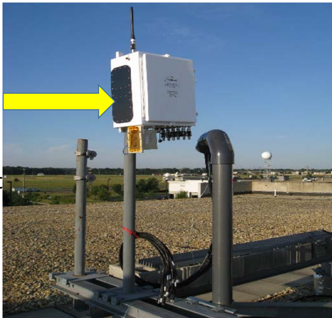
Figure 1 Photo of Tampa Microwave Emulator Installation
