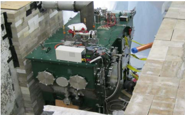
Figure 8: TDCM containing two \beta_0=0.53 prototype HWR and a solenoid during installation in the test bunker.
