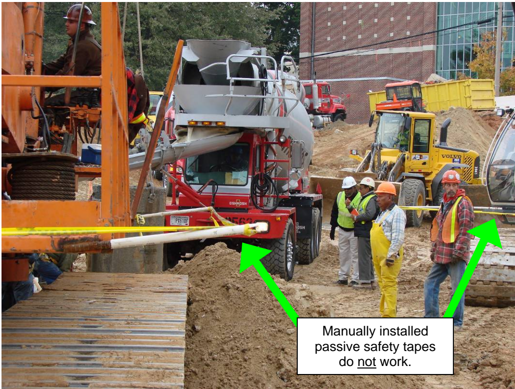
Figure 1. Currently installed best practices in safety using passive tape devices
