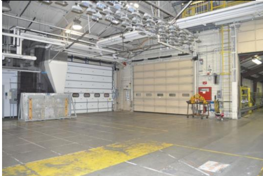
Figure 3 – Inside MPG Crash Test Building Facing South East
