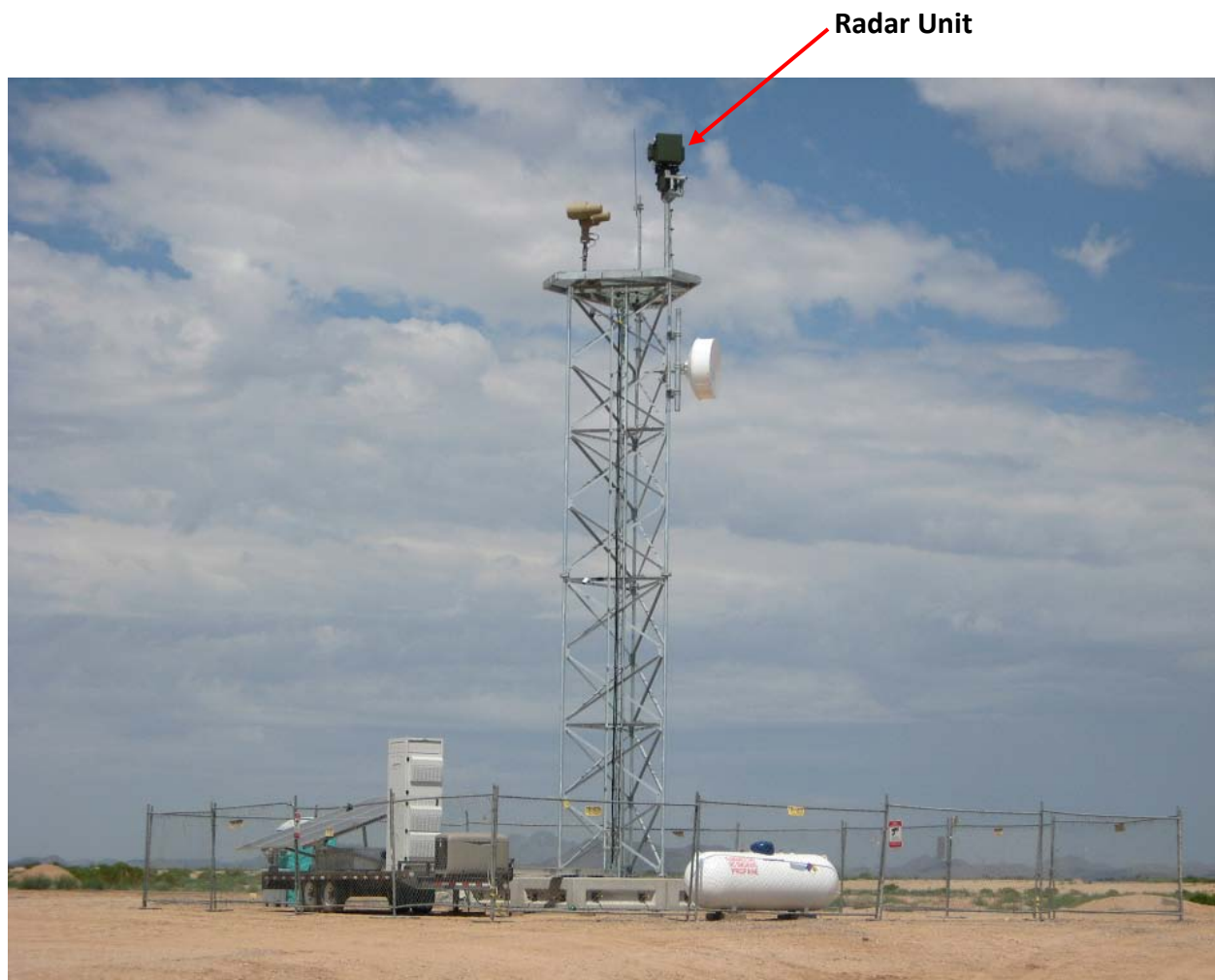
Figure 1 – Antenna Tower at Remote Site near Wittman, AZ
