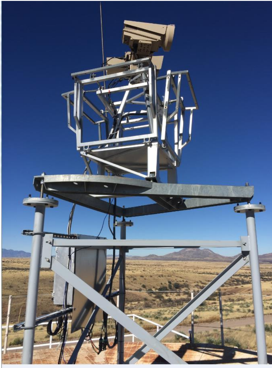
Figure 3 – Radar Mounting Structure – Fort Worth, Tx
