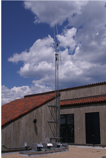
Figure 2: UHF/VHF Radio Tower
