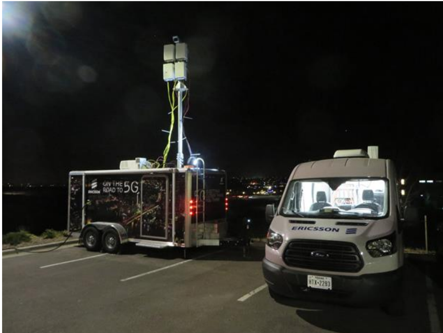
Mast and components will not extend beyond 9.2 Meters above the ground.
